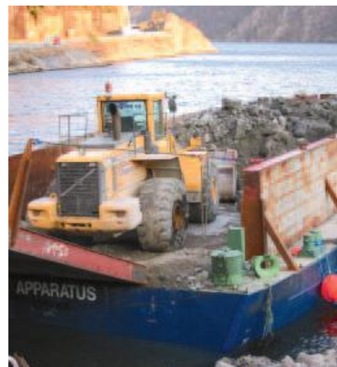
Figure 3 Use of a barge for better control of placing the rock material.
