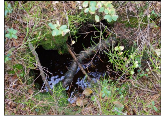
Figure 5. At location F there was significant water flow and sign that water continues eroding under the vegetation further downstream, giving it a high priority for restoration. Photo: David Arnott
